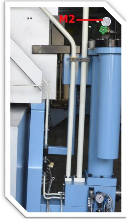
M2 AZOT BASINCI MANOMETRESİ
